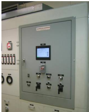
Figure 7: Example of an appended cabinet installation.
