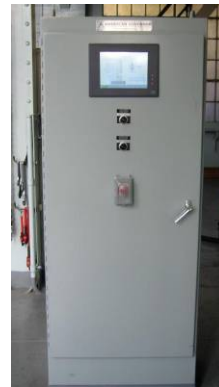
Figure 8: Example of a free standing cabinet installation.
