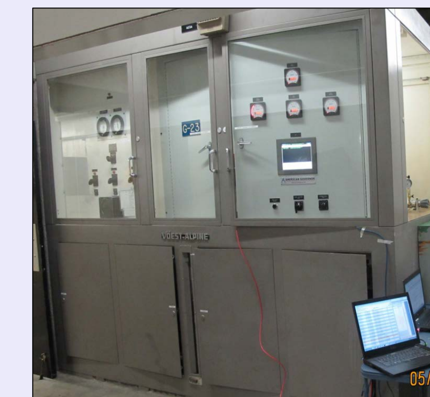
Figure 11. The Third Power Plant Unit G-23 governor, installed by American Governor Company, utilizing the Lead-Lag-Integral control scheme.
