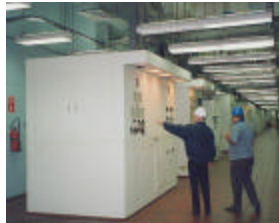
Mechanical Cabinet Actuators
