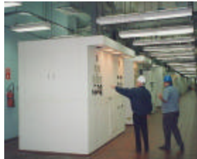
Mechanical Cabinet Actuators
