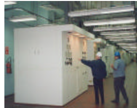
Mechanical Cabinet Actuators
