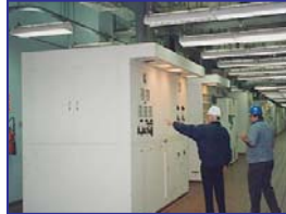
Mechanical Cabinet Actuators
