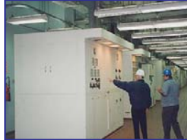
Mechanical Cabinet Actuators
