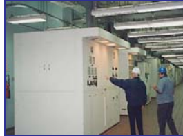
Mechanical Cabinet Actuators
