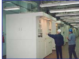
Mechanical Cabinet Actuators
