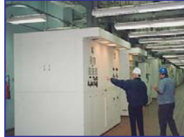
Mechanical Cabinet Actuators
