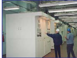
Mechanical Cabinet Actuators
