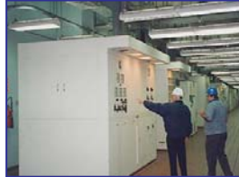
Mechanical Cabinet Actuators
