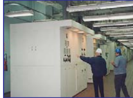
Mechanical Cabinet Actuators
