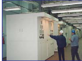
Mechanical Cabinet Actuators
